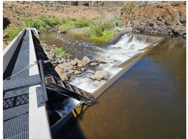
Looking downstream on Deep Creek at the O'Keefe diversion and fish ladder.
